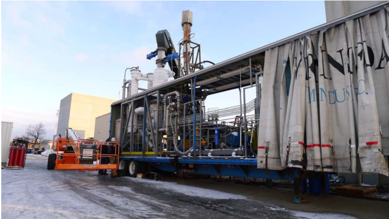
Figure 3. The completed MILS system. The GTL reactor and control room are behind the trailer curtain.
