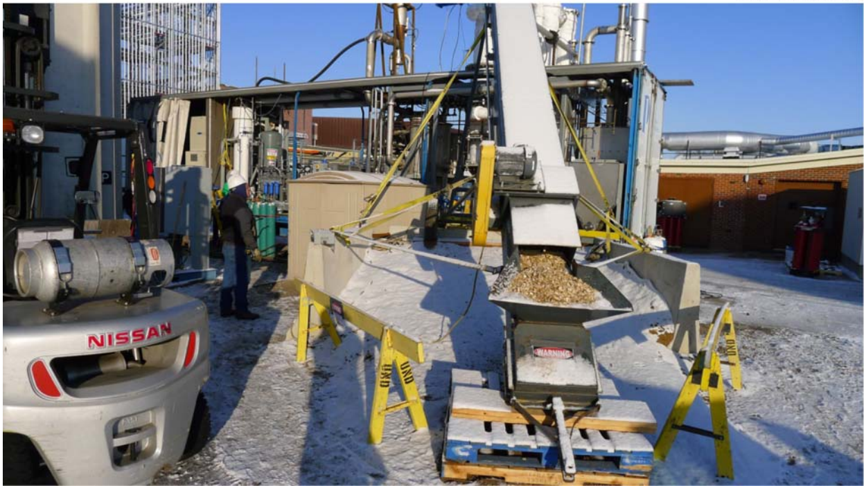
Figure 5. The conveyor used to carry the wood chips to the top of the gasifier.
